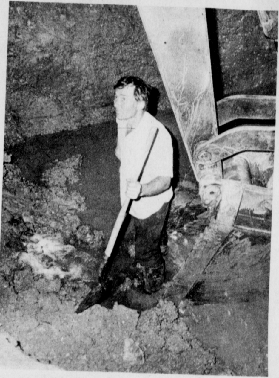
BREAK IN WATER TRANSMISSION LINE FOUND ... with help of big bucket and little shovel.
