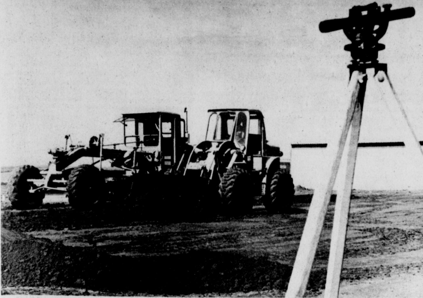
GYM CONSTRUCTION - Site preparation was underway early this week for construction of a new gymnasium at Iowa Park High School. The facility will be directly south of the present gym. Completion of the first phase is expected by mid October. Second phase will be installation of a
