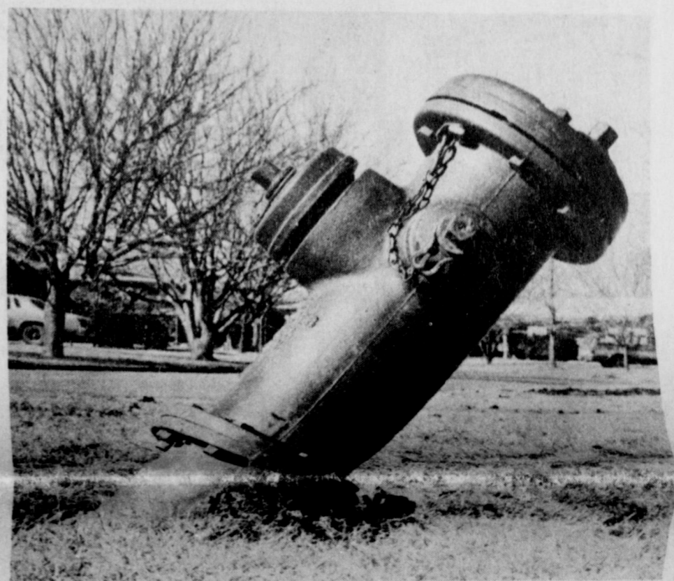
MARY'S LEANING PLUG - Mary Drive has the distinction of having a fire plug that leans more than any other in town. About 45 degrees tilt. The plug, at the corner of Douglas, apparently was knocked over by a skidding vehicle during the recent bad weather. No leaks were apparent, however, and the water department was not notified until Wednesday.
