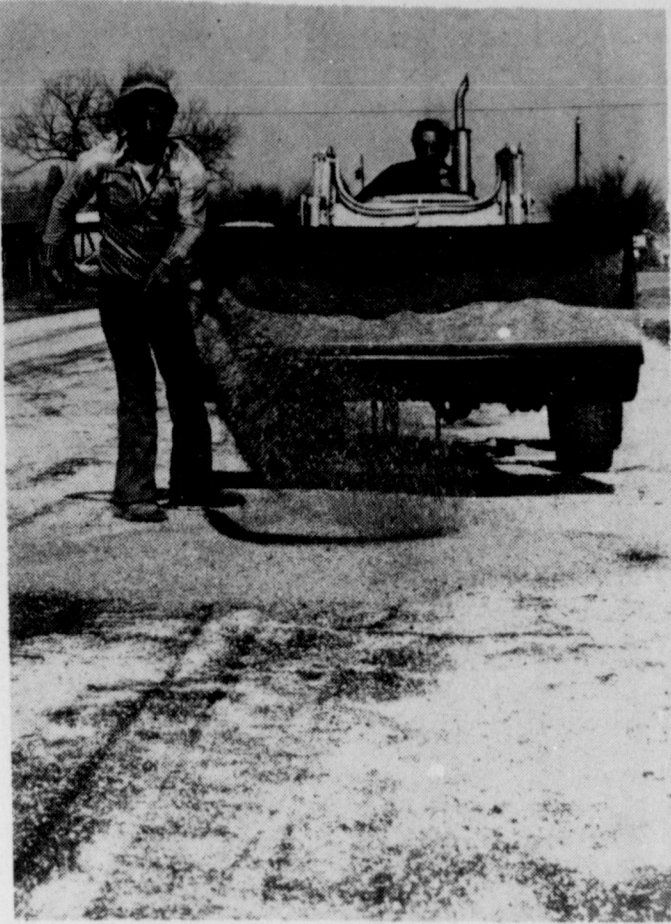
RESURFACED - Contract crews were busy this week resurfacing a portion of Bois D Arc west of Holliday Post Office. City council members Tuesday night decided to seek bids on a city-wide street improvement project.
