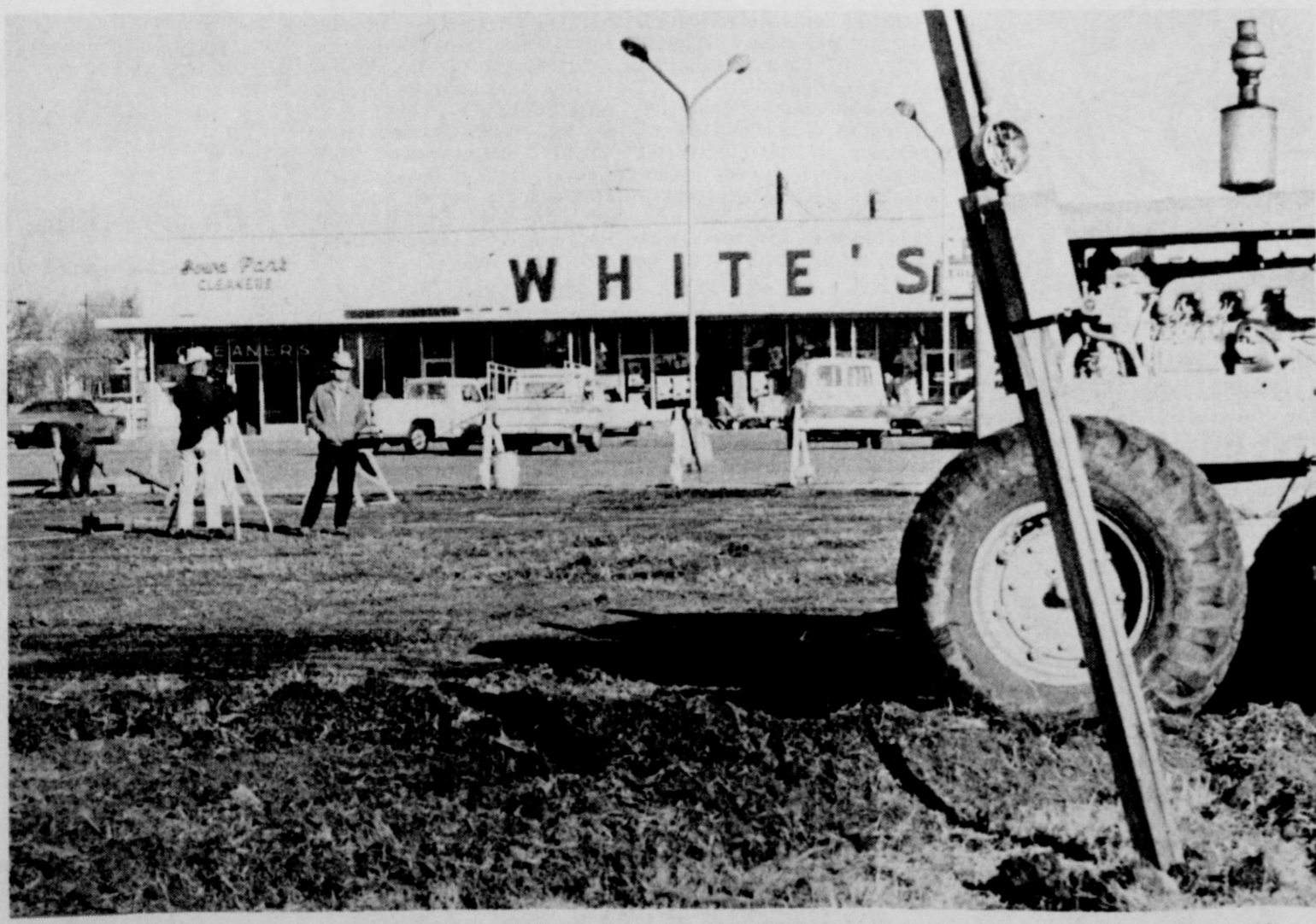
NEW BUILDING GOING UP - Workers began Monday on a new building for White's Auto Store. It is located on the south side of the Park West Shopping Center. White's has been in temporary quarters in the Center since their August fire. A block to the west the steel framework was put up this week for the new Shaw Motor Company building. And further to the west, at the intersection of Old Highway West and Johnson Road, a sign was put up Monday stating, "Future Home of Dairy Queen".
