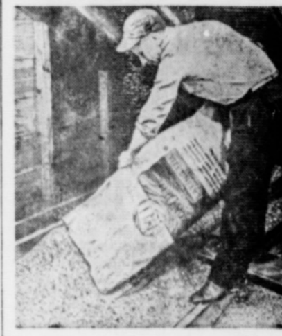
Zonolite vermiculite insulation being installed over ceiling of dairy barn at Sinissippi Farms, Oregon, Ill.
