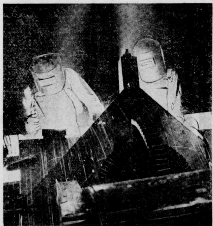
This picture is typical of the way the national defense program is progressing. Here two hooded welders at the plant of the American Car and Foundry company in Berwick, Pa., are shown at work on some of the armor plate that goes on the fighting tanks being turned out by the hundred. Tanks roll off the assembly line at a rapid rate.
