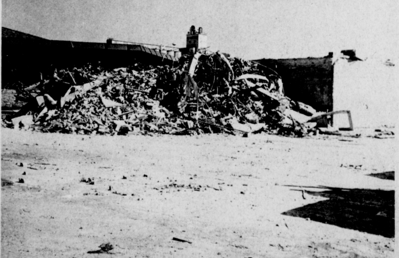
GOING, GOING..... Soon, the old First National Bank building will be just a memory. A bulldozer has piled this portion of the bank into just a pile of concrete, brick and steel. All that remains is the small portion in the background. Large trucks are moving parts of the debris of the old bank. Shown in the background is a portion of the new First National Bank building. The former bank location will become a parking lot in the near future.
