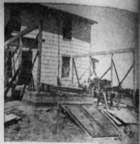
DUAL PURPOSE fallout shelter and carport-patio is shown under construction at the farm of John Holden near Hickory Grove, Mich. The shelter, to be used also for food storage, cost $1,200. With the carport and patio now being added, the cost totaled $2,300. Holden's family of three, and eight neighbors, gave the shelter a realistic workout recently when a small tornado struck nearby. An entrance to the shelter is in the foreground. (OCTOBER PHOTO)
