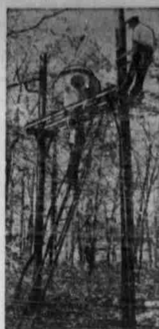
CIVIL DEFENSE siren at Winston-Salem, N. C., is installed by a fire department electrician on the Wake Forest College campus with the assistance and technical advice of Edmund F. Sullivan (on ladder), new city-county deputy CD director. Sullivan's salary is paid 50-50 by Federal and local governments as part of a nation-wide program to strengthen state and local civil defense units. (OCMD Photo)
