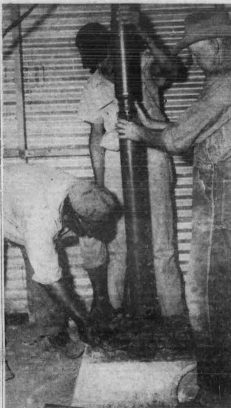
DOWN GOES WELL PUMP—A two-inch submergible pump, which will be operated by a three-horsepower motor, is being installed in one of the City of Post's water wells, one-half mile north of Close City. Since it was put into operation in 1950, the well had been equipped with a four-inch pump and a 7½-hp motor. The well tested 150 gallons per minute when it was completed seven years ago, but is now down to about 50 gallons per minute. Shown installing the pipe are Roy Maddox (right), supervisor of the well field; Pete Maddox (center), service man, and Philip Martinez, an employee of S. C. Storie Jr., from whom the City purchased the pump.—(Staff Photo).
