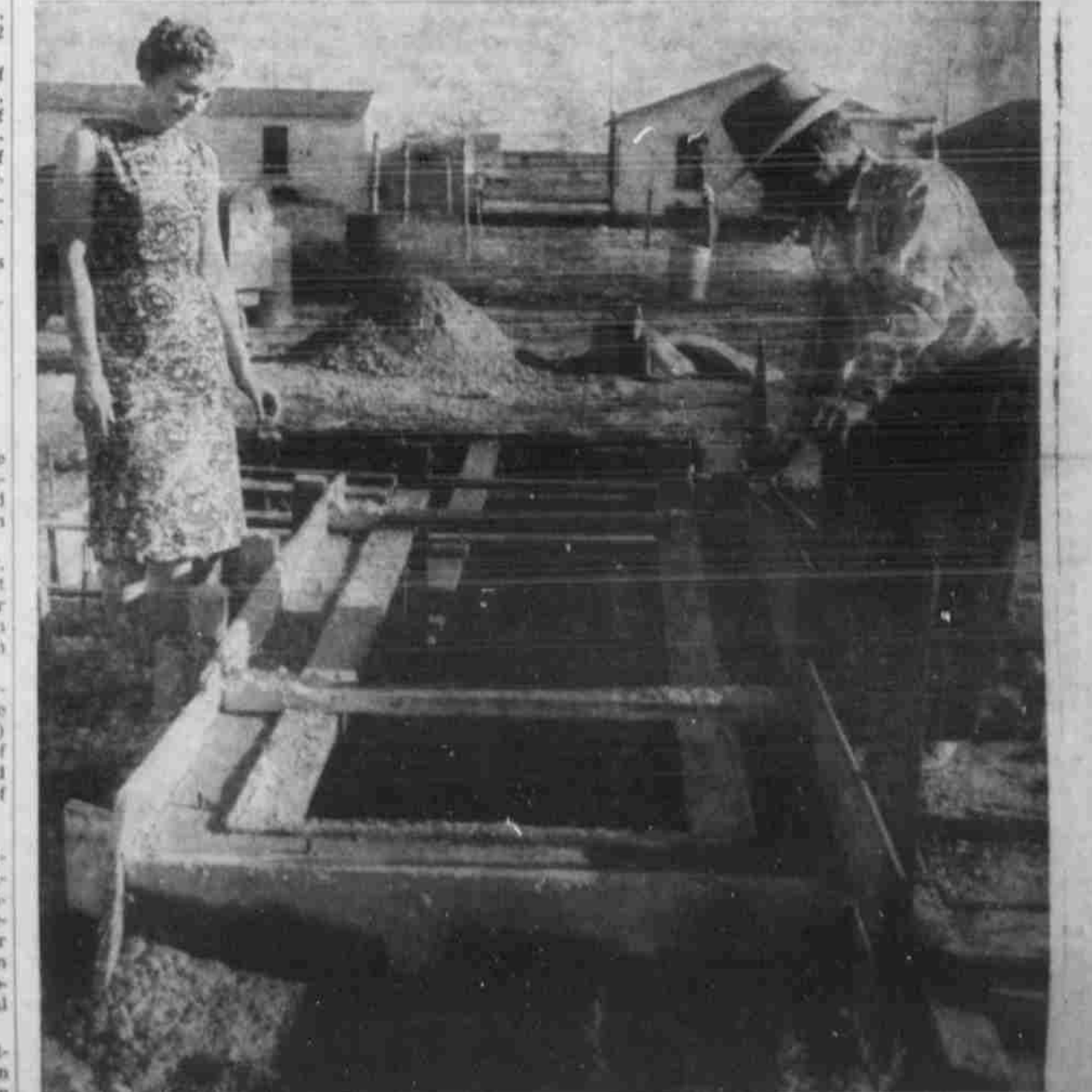
ONE OF MANY — Mr. and Mrs. Reese Carter Jr., are looking over the south corner under construction at their home at 705 West Fifth Street, one of many being built here. The Carters' cellar will be a flat-top affair, 8 by 12 and 7 1/2 feet deep. Top and floor will be of concrete and the walls of plaster. Carter plans to build a patio on the top of the cellar.—(Staff Photo).
