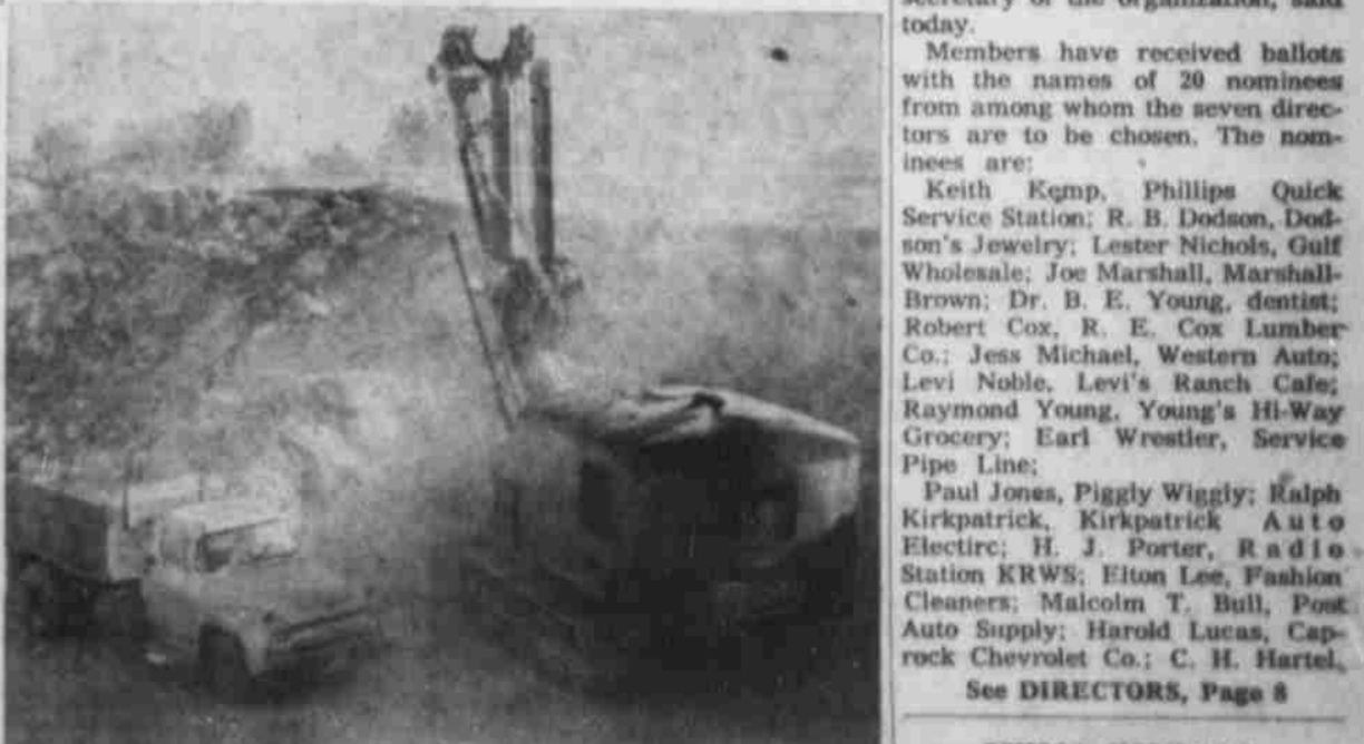
onto pit trucks and then hauled to the rock crusher at the left for processing. It then pours from the hopper into 12-cubic-yard trucks for hauling to the roadway. The pit and crusher will be in operation until the segment of the road between here and Justiceburg is completed. On the segment between Justiceburg and the Scurry County line, a rock pit near Fluvanna will be used.—(Staff Photos).
