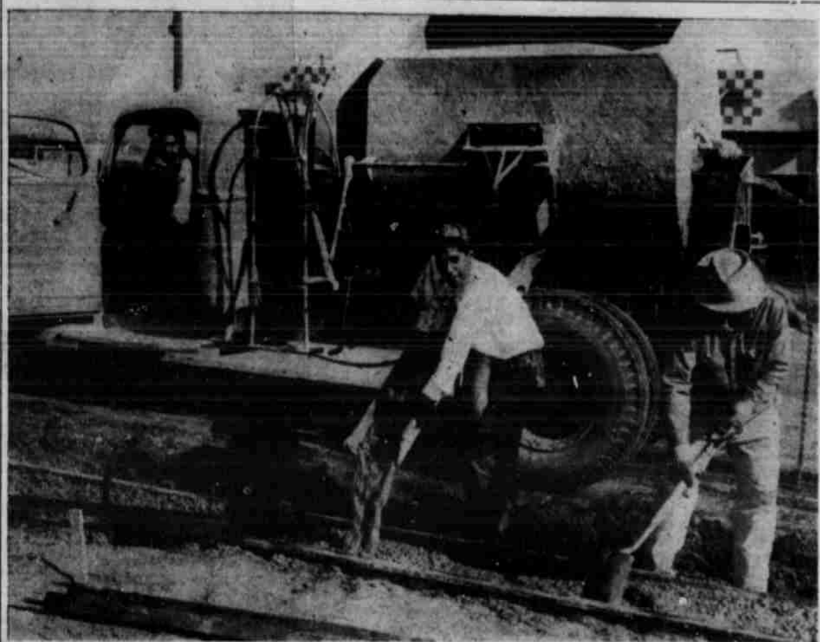
WORK BEGUN ON HIGHWAYS — Pictured above is a crew working on the curb and gutter for the initial step on the highway widening project slated here. The crew is part of Bob Phillips' construction crew which began on the project Monday morning after some two months of delay and postponement due to weather and previous engagements. (Photo By Dispatch Photographer)
