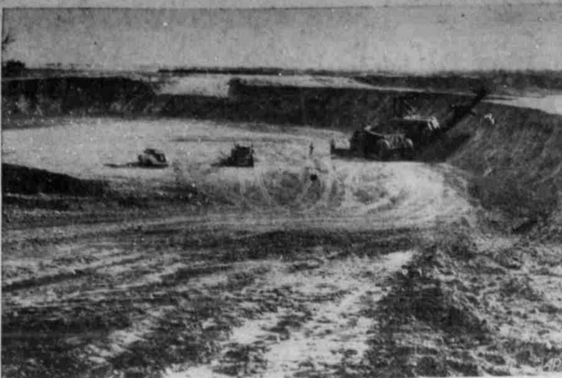
FALCON DAM PROGRESSES — Earth moving machines continue work on the international Falcon Dam being constructed in the Lower Rio Grande near McAllen. Except for spillways and power plants in the river bed, the five-mile long structure is earthen.
