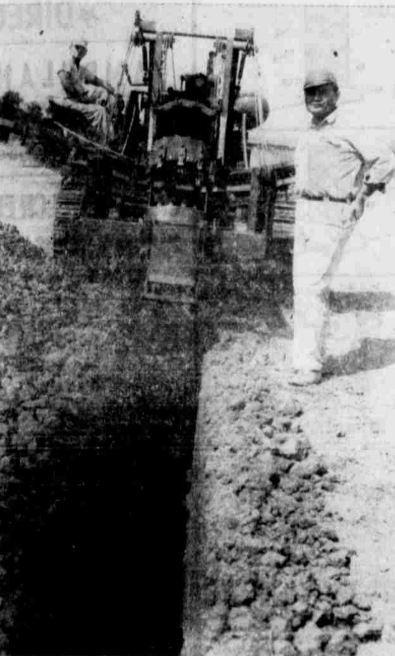
JUST GETTING STARTED Laying of 8-inch cast-iron water pipe in the extreme north-west of town was just getting under way when this picture was taken. At the right is Walter Ellerd of Lubbock, contractor, and on the ditch-digger is Frank Lewis.—(Staff Photo.)
