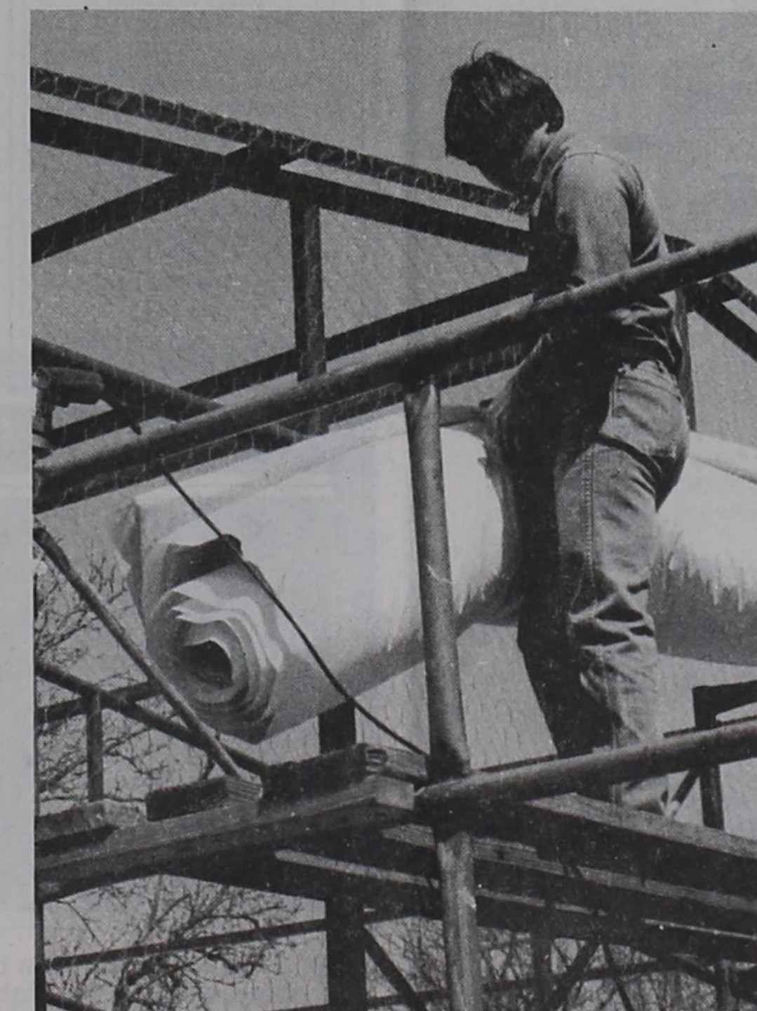
COTTON INSULATION is getting special attention in this area as builders and contractors discover the special advantages of the product. Guinn Miller installs vinyl backed cotton insulation on a metal building being constructed in Post. He and Fiber-Cell Insulation Inc. owners David Woods and Sammie Palmer expect to sell up to six million square feet of the product this year. They are distributors for cotton insulation materials manufactured by Cotton Unlimited, Inc. The cotton insulation has recently received a certification of approval by the Texas State Board of Insurance. "We will be offering attic blow in insulation in the near future," Palmer reports.
