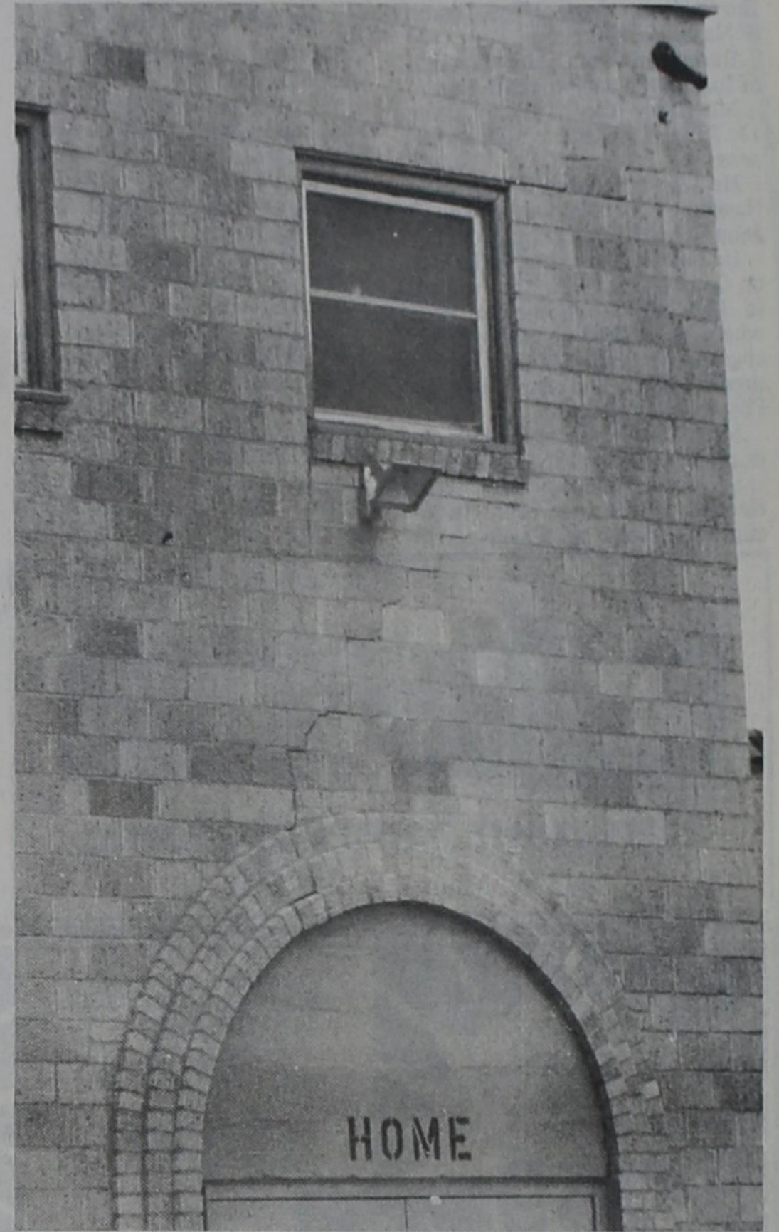
CRACKS in the walls of the old junior high gymnasium have doomed the 50 year old structure for demolition.
