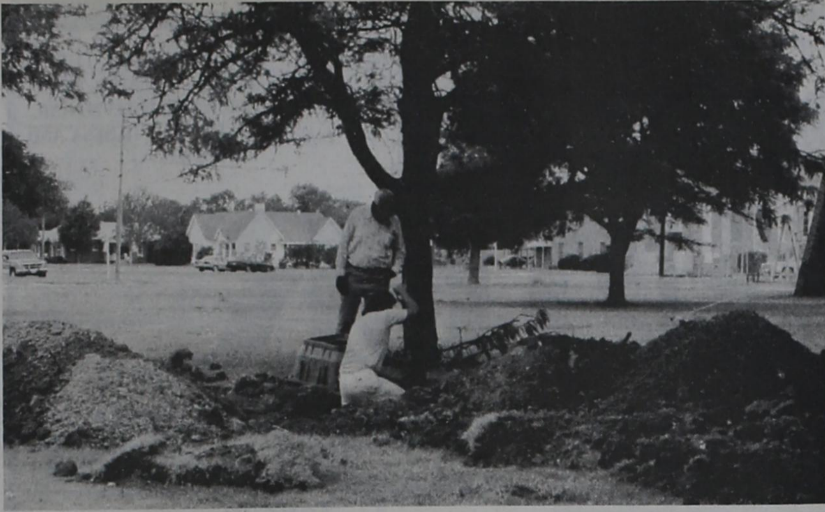
CITY EMPLOYEES are installing a water line to service a fire hydrant to be placed at the southeast corner of the courthouse. The new line will also serve the new West Main Street landscaping project. (Photo by Becky Warren)
