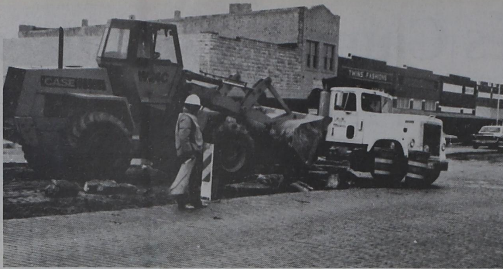
GETTING READY TO PLANT TREES - Construction crews from H & M Dirt Contractors removed the old asphalt and leveled three blocks on East Main Street in preparation for the landscaping project.
