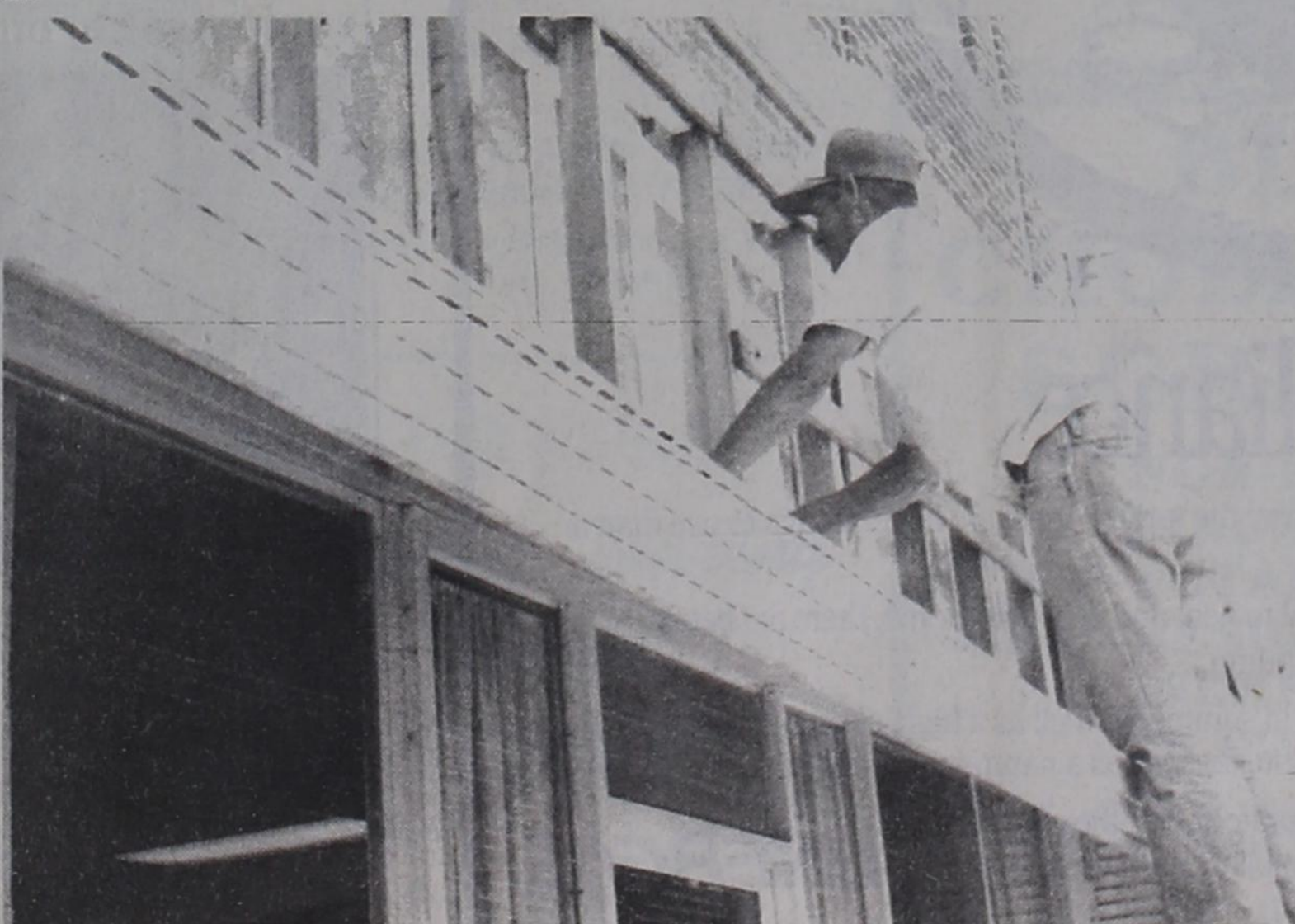
MASONIC LODGE RENOVATIONS - Scott Davis begins work on the facade of the Masonic Lodge on North Avenue I in Post as the building undergoes a renovation project that involves removing the aluminum slipcover, replacing broken windows and painting the wood trim and awning. The project is due in part to a grant from the E.A. Franklin Trust and the Main Street Project. Also working on the renovation, but not shown, is Floyd Davis.
