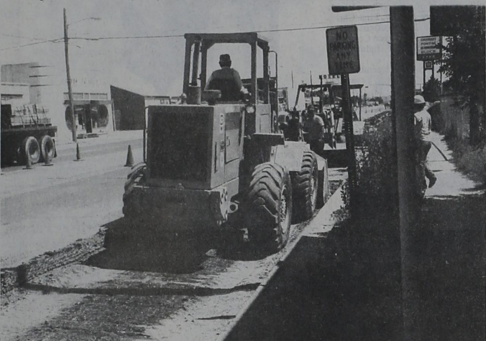
HIGHWAY DEPARTMENT AT WORK - Construction equipment moved into Post as the Texas State Highway Department began work preparing U.S. Highway 84 for a six-inch overlay, as well as routine maintenance of the highway. The construction revived rumors of a highway to go around or to bypass Post, but these rumors were quickly laid to rest by City Manager Bob Turner who was assured, when talking with the District Highway Department and the Planning Department in Austin, that there were no plans - immediate or long-range - to build a highway around Post.
