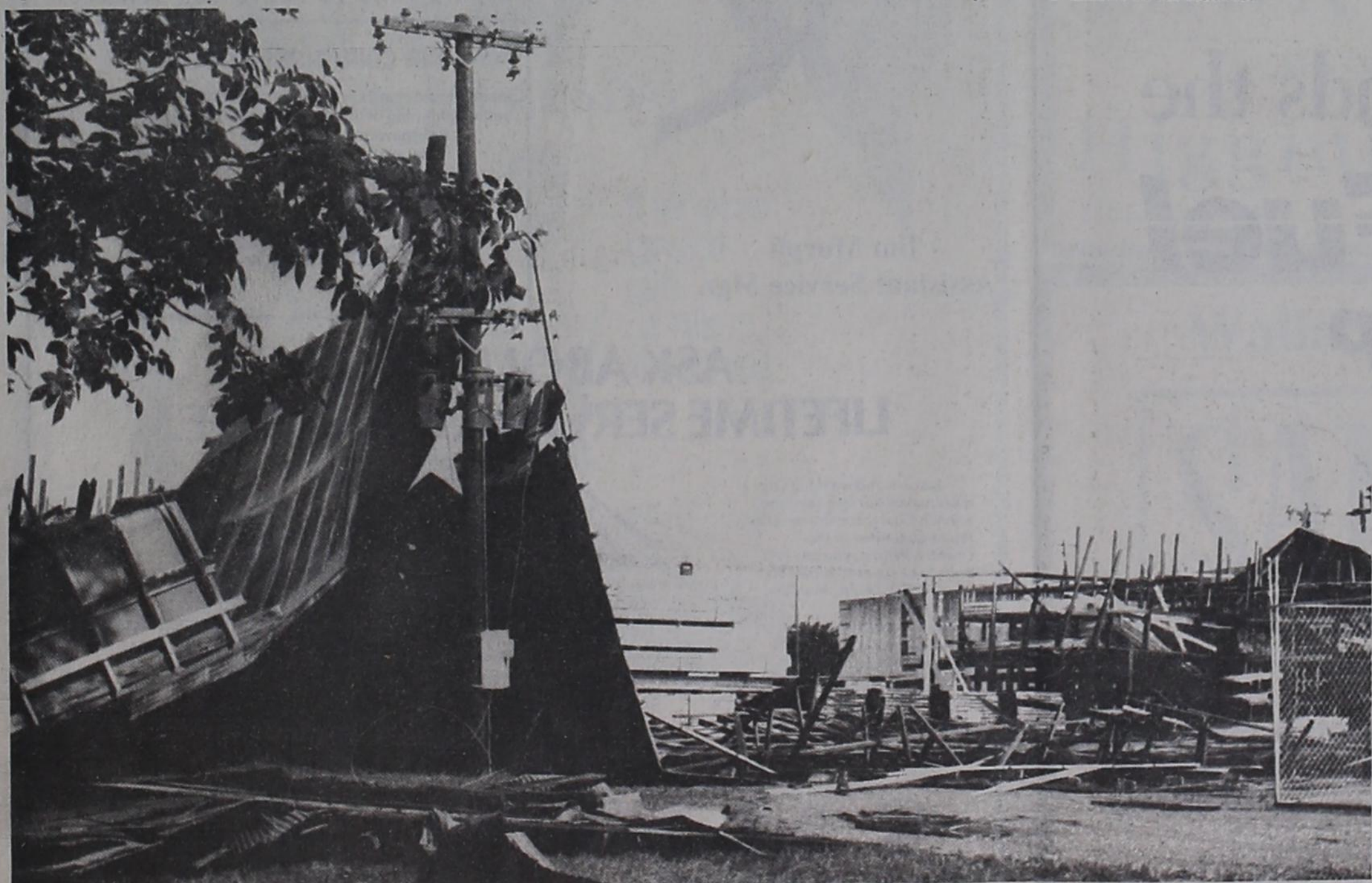
DESTRUCTIVE WINDS ripped through one of the main storage barns at Higginbotham-Bartlett late last Thursday afternoon, which resulted in the loss of electric power in the downtown area for several hours.
