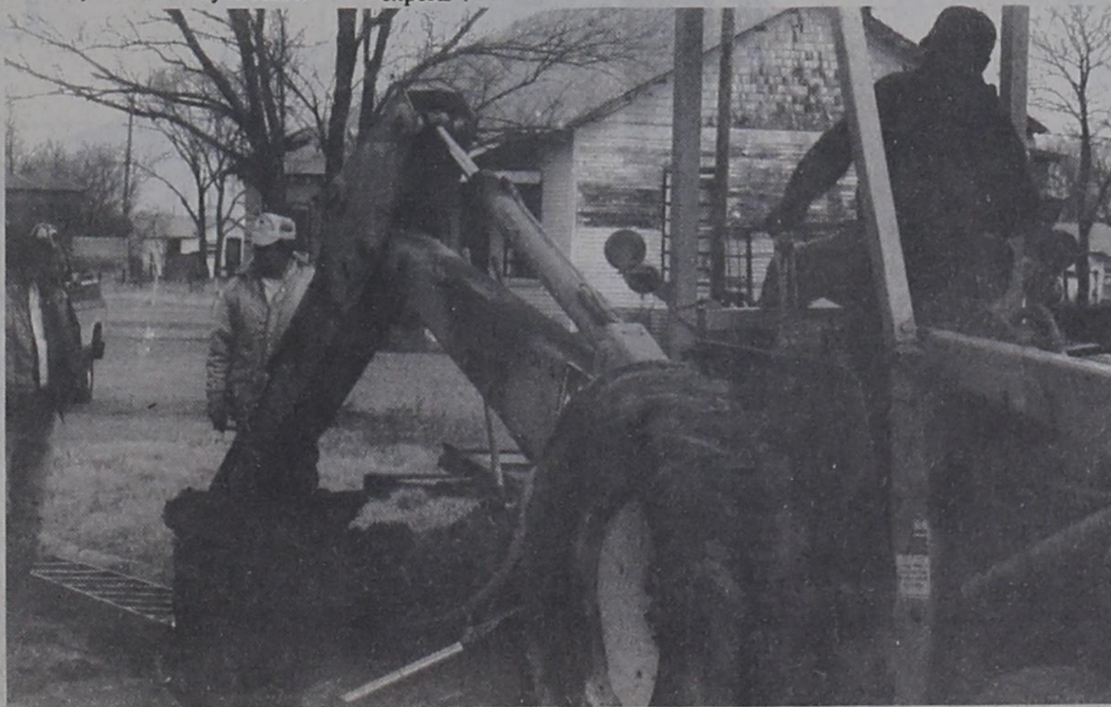
CITY AND WHITE RIVER maintenance crews work to repair a leak in the main water line into Post last week. The leak did not affect service to the city and was repaired within a few hours.
