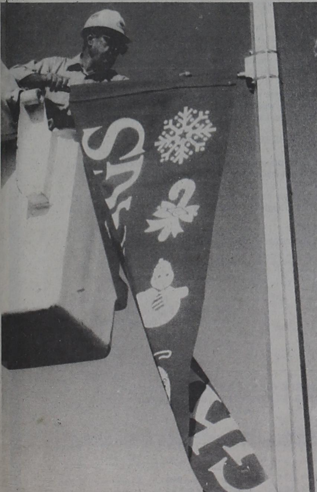
NEW HOLIDAY BANNERS - Southwestern Public Service's Jimmy Baker installs a sample of a new holiday decoration being considered by the Post Main Street Project, Post Chamber of Commerce and Post Merchants' Association. Public opinion of the banner idea is being solicited by the three organizations. The banner may be seen on East Main Street. Changing to the banners will depend largely on public opinion. Post residents are encouraged to call the Chamber of Commerce at 495-3641 or the Post Main Street office at 495-4157 to express opinions. If approved, banners for various holidays and special occasions could be installed, using the permanent brackets on utility poles.
