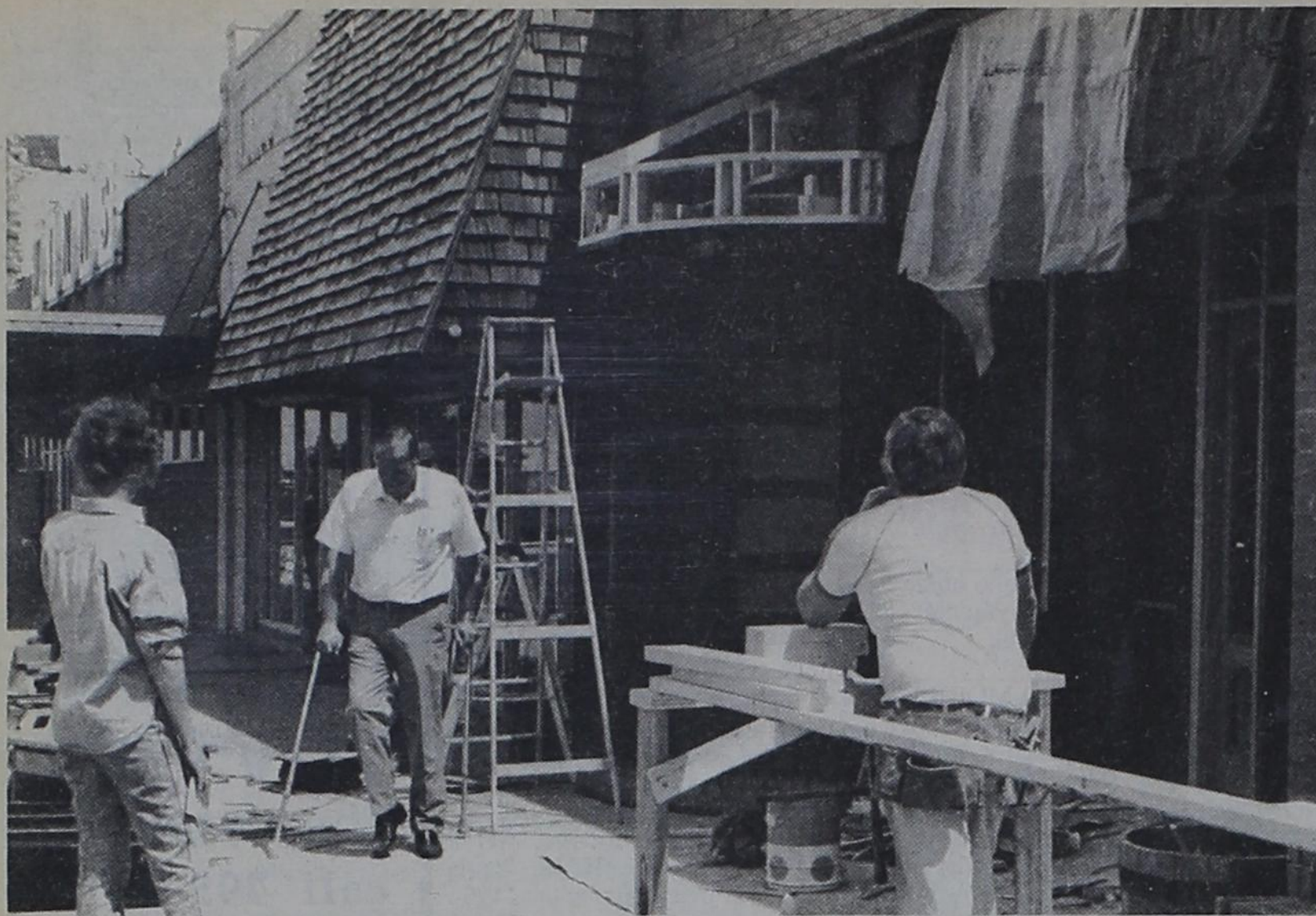
MAIN STREET RENOVATION - Jan Crawford (left) inspects the remodeling of her store, Jan's, and the construction work being done on Manna Square, a new addition to downtown Post. Manna Square, a number of specialty shops under one roof is scheduled to open soon.
