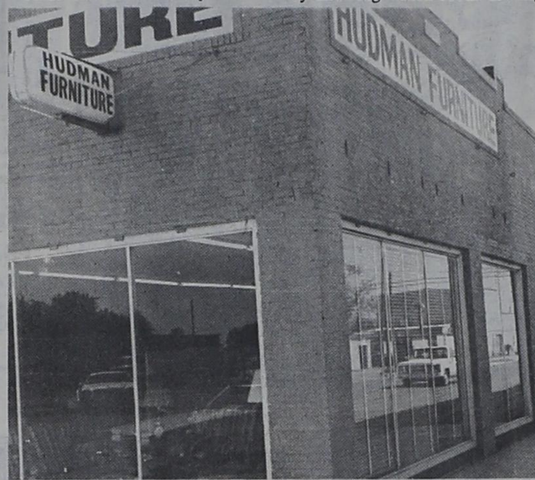
IMPROVEMENTS DOWNTOWN - Project Mainstreet renovations continue, as evidenced by work at Hudman Furniture on East Main Street.
