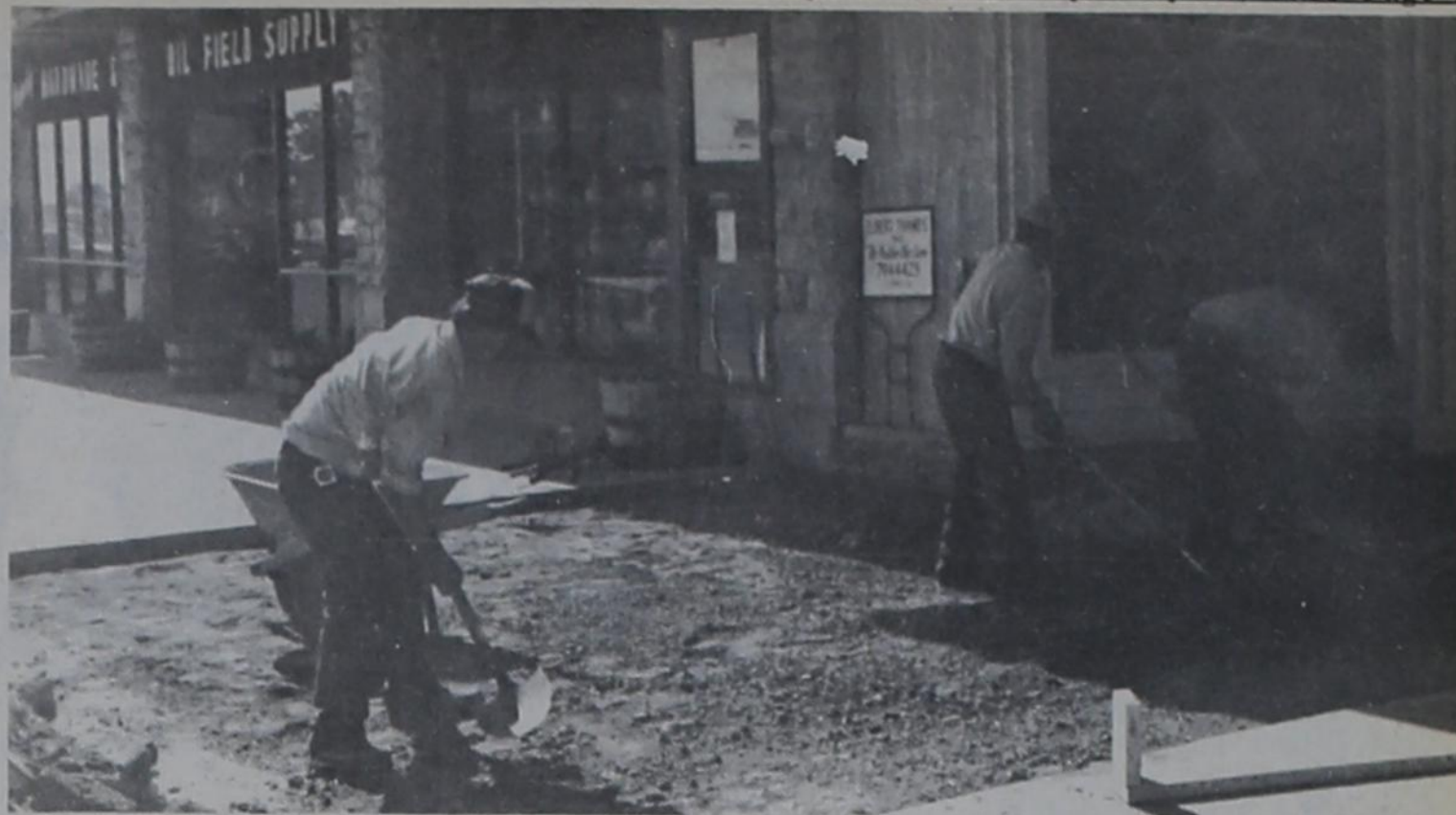
MORE IMPROVEMENTS DOWNTOWN - Construction crews continue remodeling and expansion work at Handy Hardware on East Main Street.
