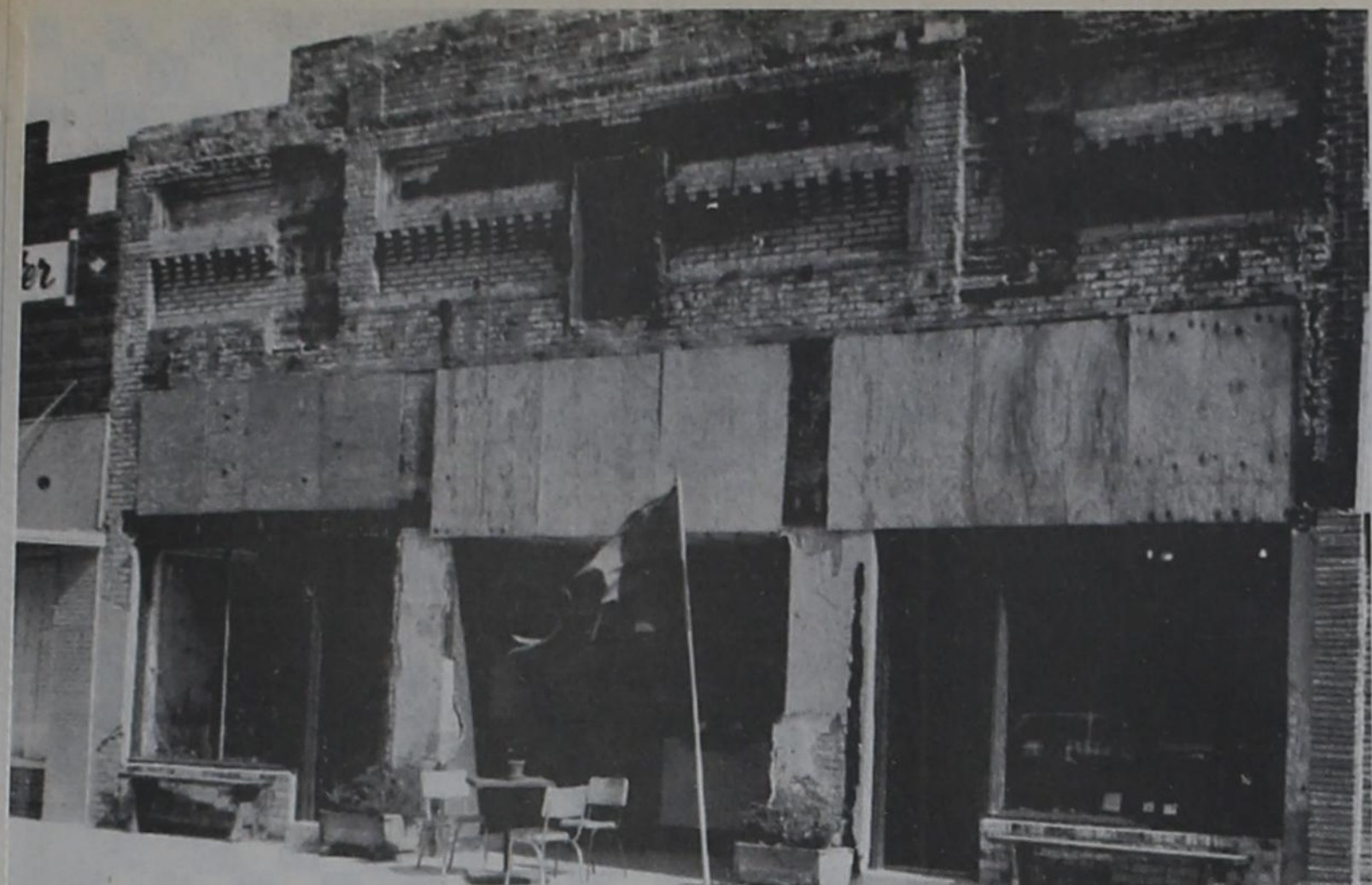
THE ORIGINAL Palace Theatre building shows the weathered wear and years of changes following removal of stucco. Now housing the Garza Theatre, the building was constructed in 1916, according to the raised lettering high faintly shows in the middle top. Due to the serious deterioration of the brick and the destruction from previous work of the brick, plans now call for replacing the stucco and repairing door and window trims.
