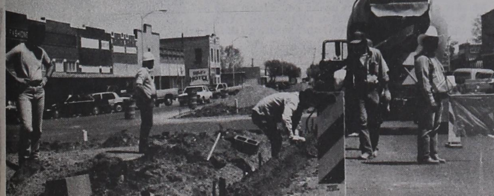
PUTTING IN THE CURBS has been the order of business the past week as the East Main Street landscaping project begins to take shape. Trees are expected to be planted next week.
