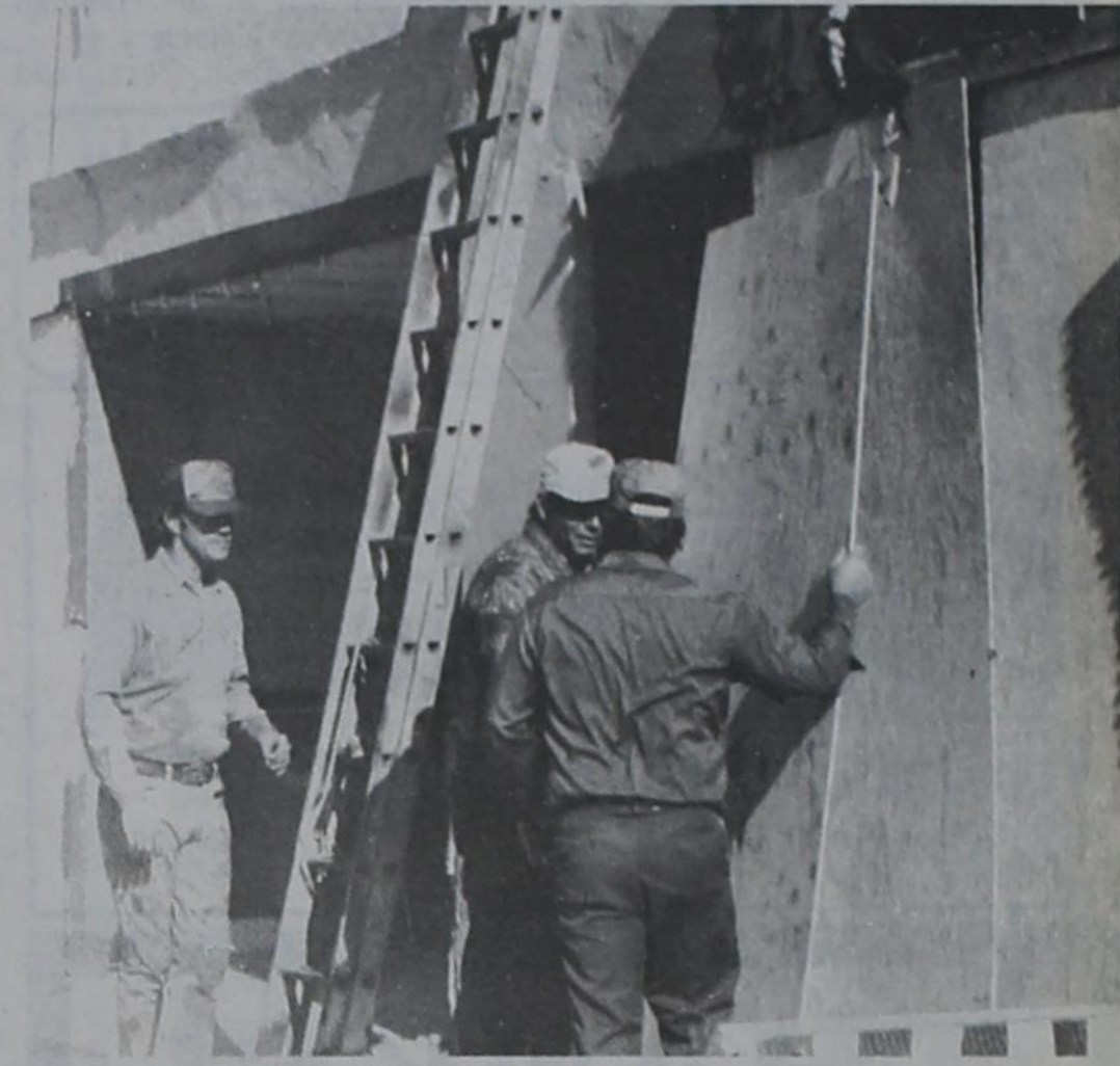
CONSTRUCTION began last week on renovating the front of the Garza Theatre. New stucco will be applied to the front in a remodeling project made possible by a Post-Montgomery estate contribution.
