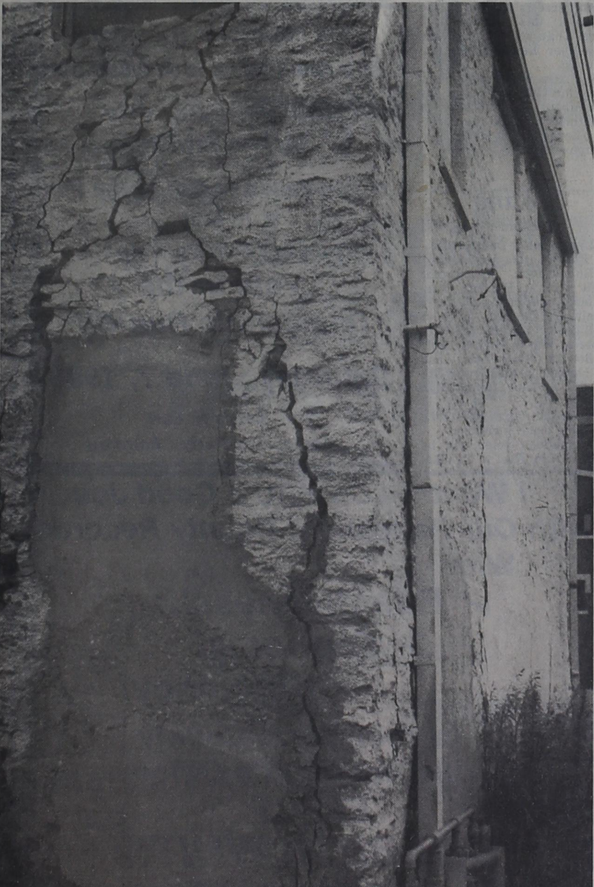
A WALL ABOUT TO COLLAPSE is the way engineers describe the south and west walls of the Algerita building downtown. Efforts are underway by the Heritage Association to raise funds to save the building.
