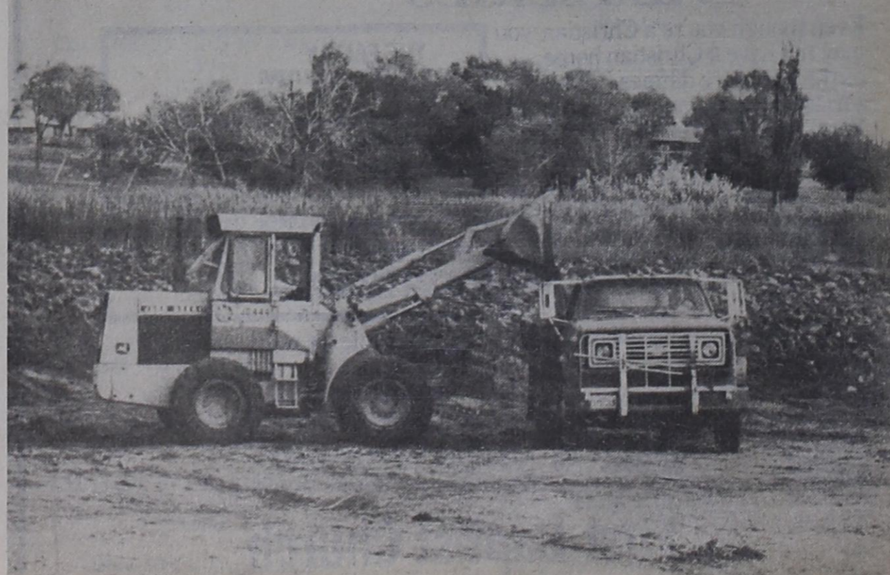
SOUTH LAKE FACELIFT — The city and county are combining their resources to dredge the sides of South Lake while the lake is down. All available equipment was in use this week with visible progress being made on the project.
