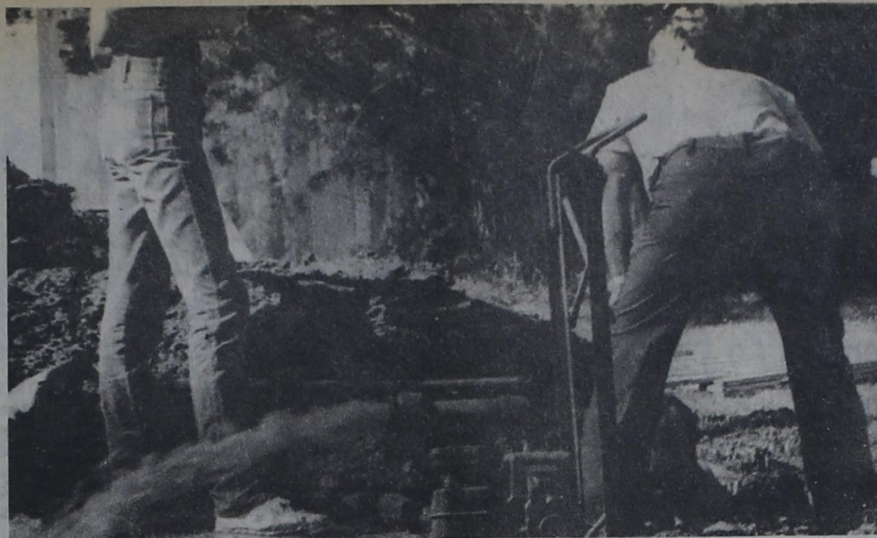
REPAIRING WATER LINE — City workers caused a minor flood down Broadway Saturday morning when they were repairing a line on West 12th Street.
