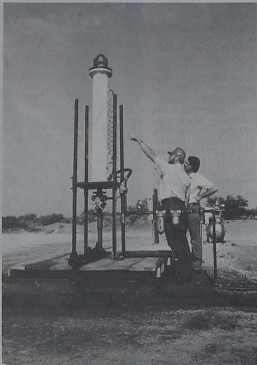
FIRST INSTALLATION — The first pneumatic pump to be installed in the Permian Basin was on this HNG Oil Co. well near Jal, N.M.
