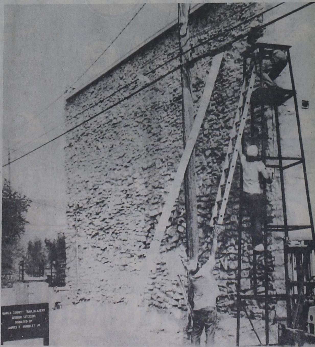
SAVING THE ALGERITA - Jerry Osborn and his crew put the finishing touches to the recently repaired south end of the Algerita building. Osborn donated his time and the cinder blocks, saving the Garza County Heritage Association approximately $23,000.
