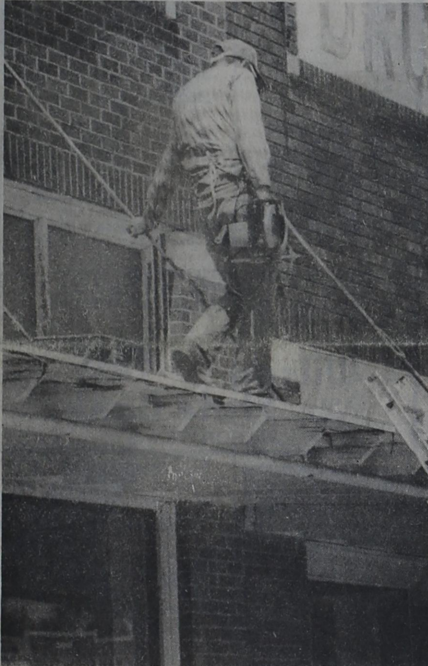
FRONT GETS REPAIR - Work on repairing and renovating the front of Western Auto helps put a
