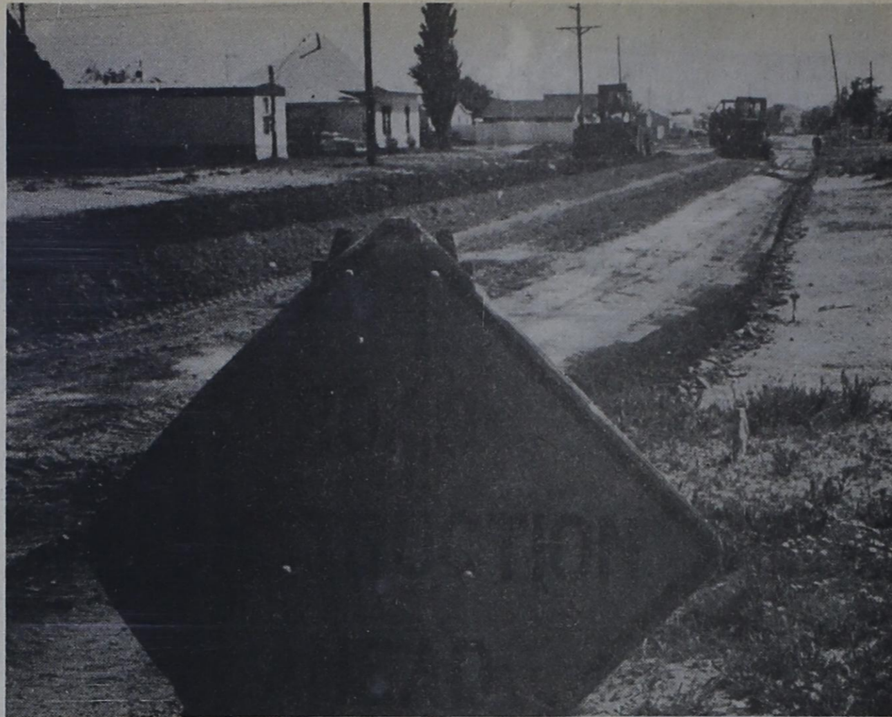
PAVING BEGINS - The 1984 city of Post paving project began this week, with Avenue I near the football stadium getting attention from the construction crews.
