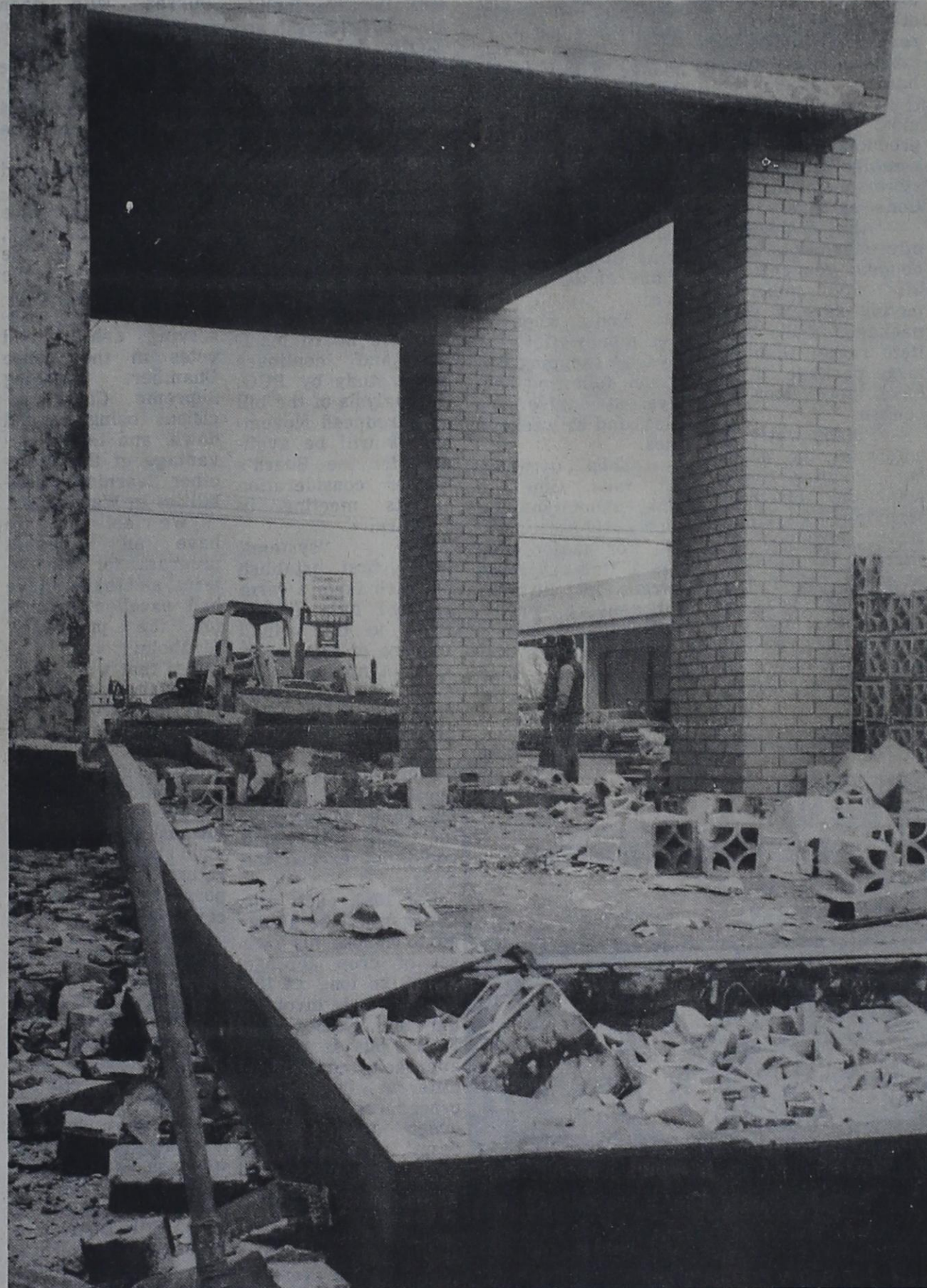
The finished product will be worth all the trouble, as the Post City Hall restoration work starts showing outward signs of progress. At the current rate, construction is expected to be completed on the renovation work by late spring. (Photo by Tim Burnett)
