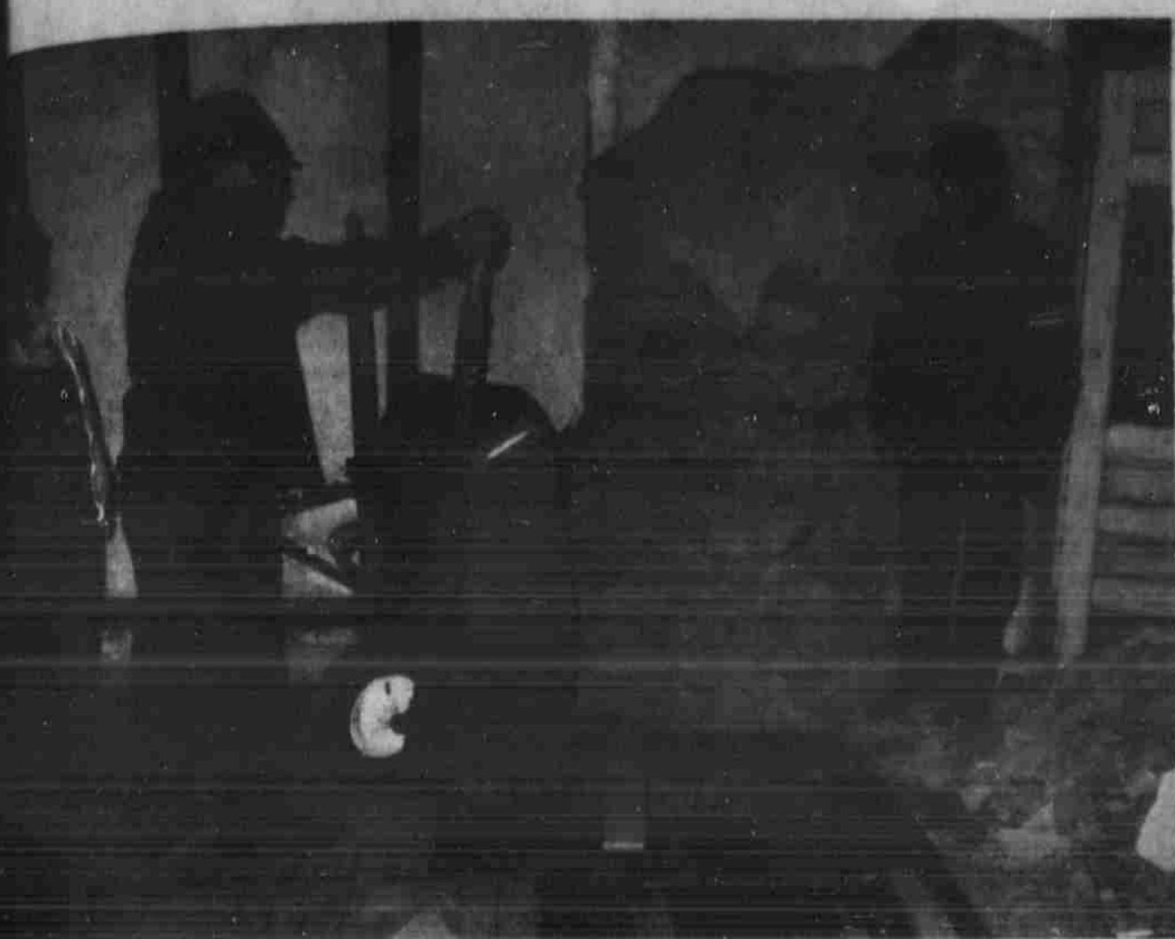
URING SUPPORT BASE — David Newby, left, supervises the pouring of cement bases at the rear of the Algerita Hotel on which will be erected pipe supports for the heavy wooden trusses to take the weight of the trusses off the brick wall. It was this weight which caused the brick wall to buckle. Dumping the cement is
