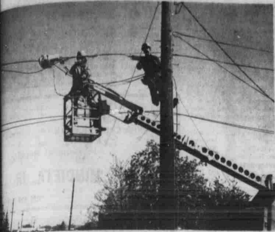
INSTALLING NEW PHONE CABLE — General Telephone linesmen, Perry Dietrick and Mark Taylor, are shown above placing new phone cable in Post.
