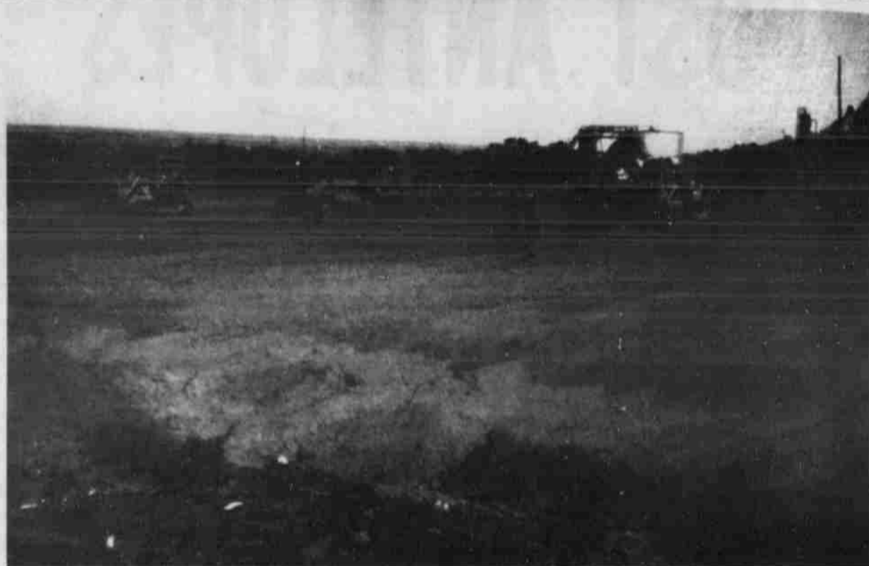
PREPARING NEW DRILLING SITE — Four pieces of H&M Construction equipment prepare a new drilling site for the George R. Brown oil interest just south of Post.
