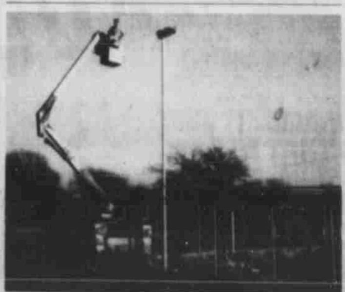
LIGHTS GOING UP — Richard Dudley is shown above installing lights for the now-under-construction tennis courts in city-county park which the city is building in the area east of the barbecue tables at the south end. — (Staff Photo)
