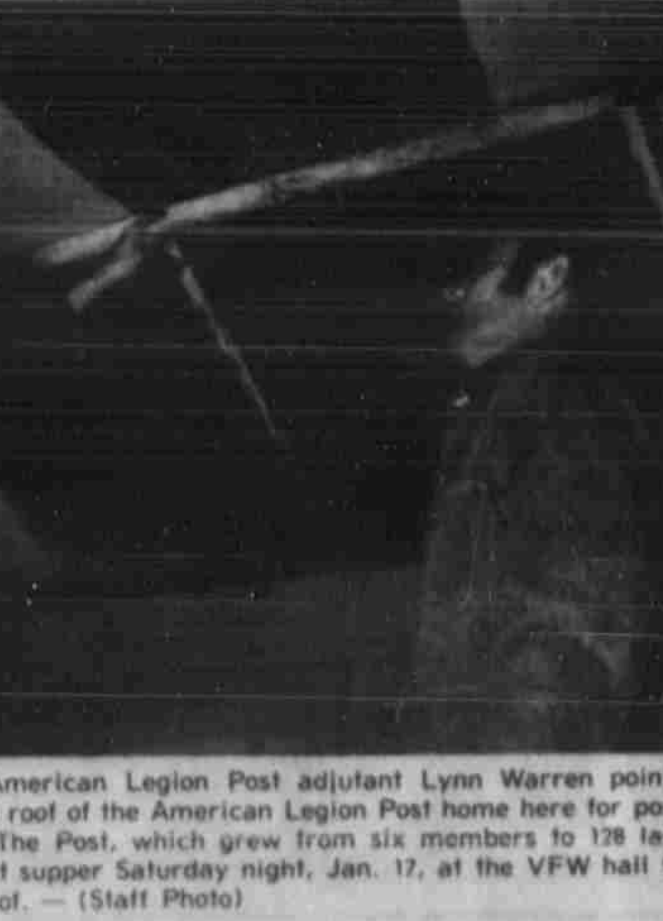
A ROOF IN NEED — American Legion Post adjutant Lynn Warren points through ceiling to holes in roof of the American Legion Post home here for post commander Archie Gill. The Post, which grew from six members to 128 last year, is planning a benefit supper Saturday night, Jan. 17, at the VFW hall to raise money for a new roof. — (Staff Photo)
