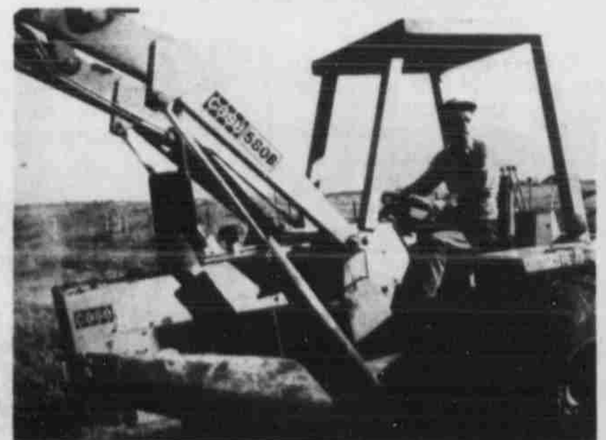
JIM MASON, backhoe operator, building a tank pad on the Edwin L. Cox lease.
