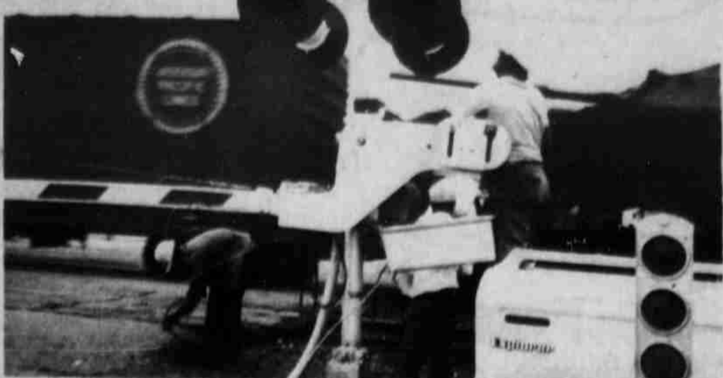
FOR SAFETY'S SAKE — R. Dillon of Slaton stands in the back of a pickup to check the new crossing gate's operation at the West Main Street crossing as a train roars through. Just above the workman stooping at the left can be seen one of the four crossing gate arms, which went down 29 seconds before the train reached the crossing. — (Staff Photo)
