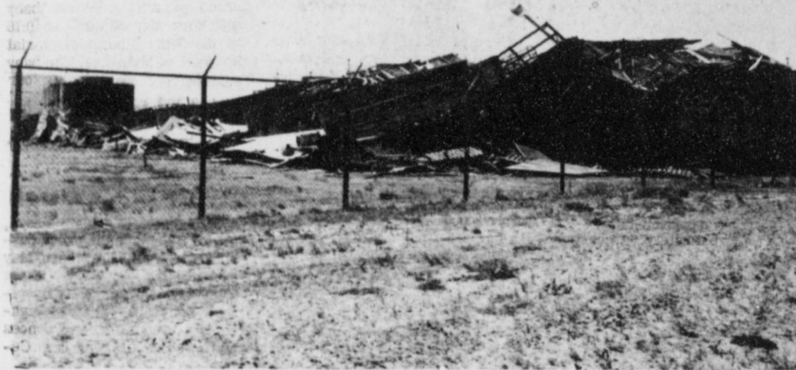
WIND DOES DAMAGE AT PLANT X... Evidently, a very strong wind did this damage to a cooling tower at Plant X Tuesday afternoon. Bob Drake, plant manager, reported that the strong winds blew down this cooling tower. There were no interruptions of electrical power due to the damage. He reported that it will be several weeks before the cooling tower can be repaired and that he had no idea of the amount of damage, money-wise, the plant sustained.
