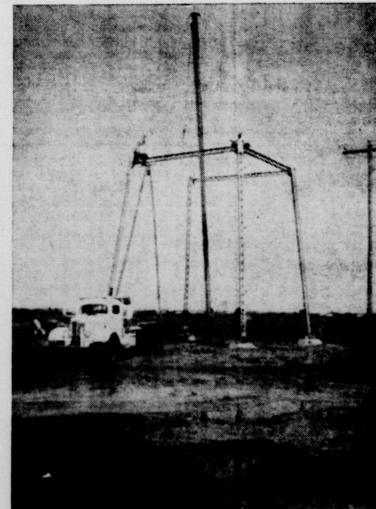
THALIA WATER TOWER GOING UP—Shown above is the new water tower for Thalia's new water system that is being built just west of town. This picture was taken last Friday afternoon, and the workers are shown in the upper portion of the picture as they assembled the tower.
