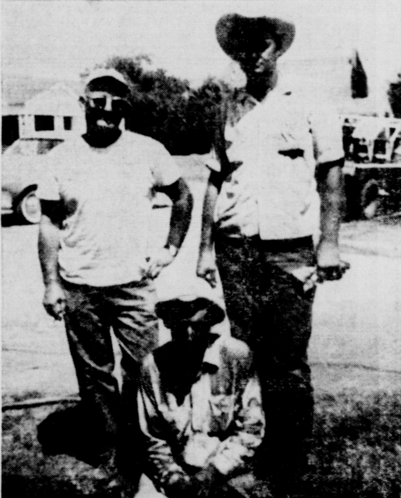
While the water department men were on North Third, the Texas Natural Gas Co. employees, Charles Branch, Buster Dishman and Lester Dockins, kneeling, were found on North Second repairing a gas main. To all of these men and their helpers, we say "thank you." We appreciate your services.
