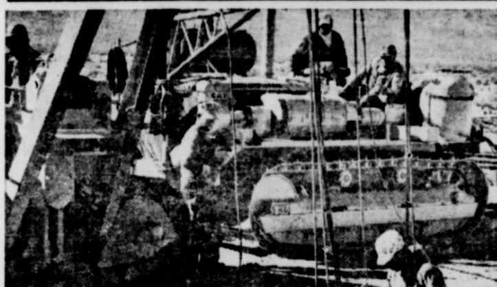
WORKMEN are hurrying to completion a new 34" pipeline from the Arizona border 116 miles to Newberry, Calif., to provide increased natural gas for the Southern California basin. (CNS Photo)
