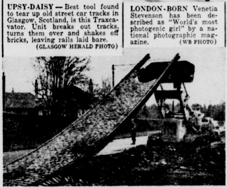
UPSY-DAISY —Best tool found to tear up old street car tracks in Glasgow, Scotland, is this Traxxator. Unit breaks out tracks, turns them over and shakes off bricks, leaving rails laid bare. (GLASGOW HERALD PHOTO)
