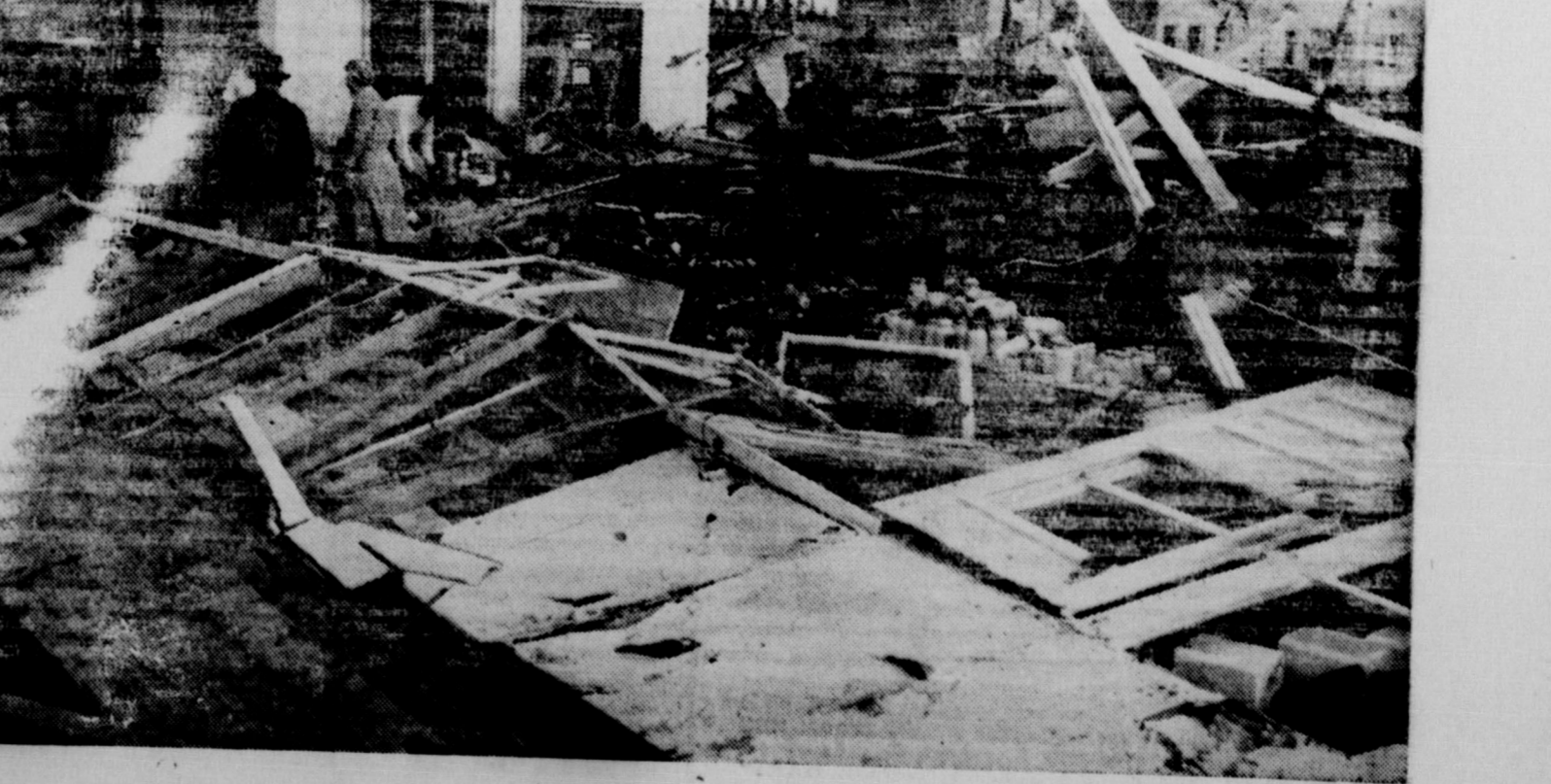
Foodstuffs were laid open to the elements in Crowell's tornado. Here is a view of a grocery store after the twister struck. While the building was wrecked, many of the glass containers were not damaged. J. L. Brooks, store owner, is shown seated on the wreckage in the center. He offered to trade the store for a camera.
