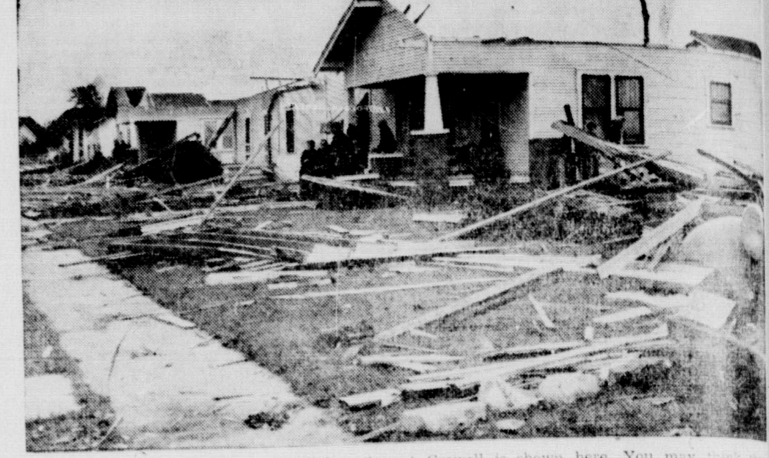
Part of the storm ridden residential section at Crowell is shown here. You may think buildings were badly damaged, as they were, but they escaped lightly compared with the homes that were blown to bits.
